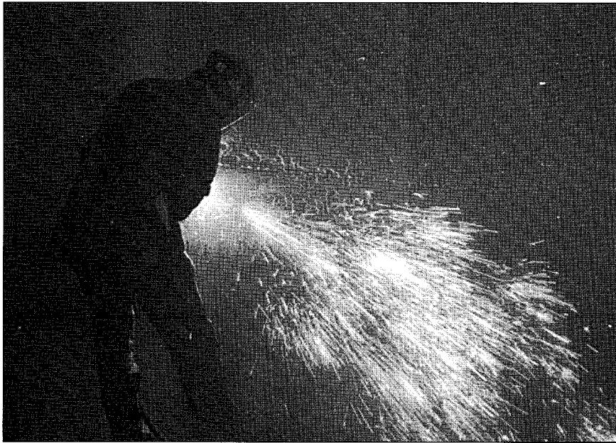
Welder shielded-metal-arc-welds a filler-metal deposit to fill pits of a steel water tank.
